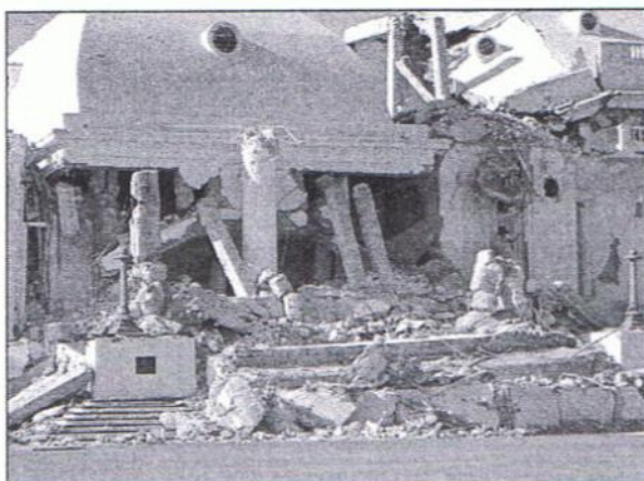
The Presidential Palace suffered the same fate as most other buildings in Port-au-Prince.
