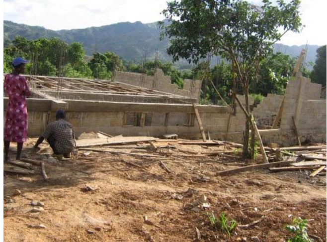
Christ the King School in Cotelette, Haiti, currently under construction – completion scheduled 06/06.
